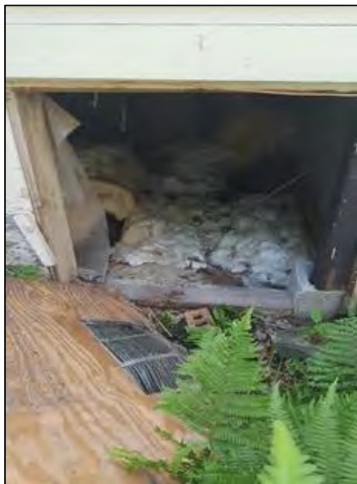
Photo 2: Behind the loose panel under Dawn’s building
